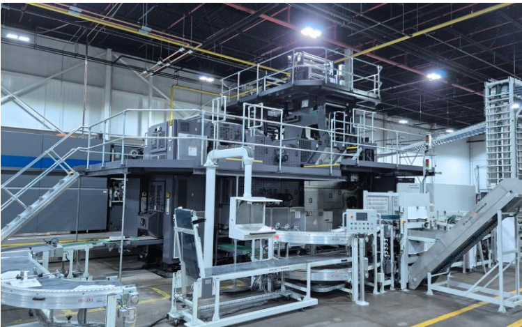
Image 2 shows: highly flexible PFC-252 pin folder by manroland Goss during the installation phase at Lakeside Book Company in Willard, Ohio
